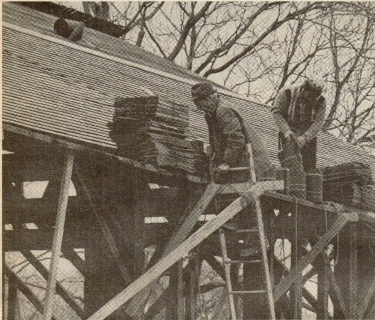
When the weather is nice, workmen continue to assemble, piece by piece, jig-saw fashion, the barn that is going up on the old Riverdale Zoo site.
