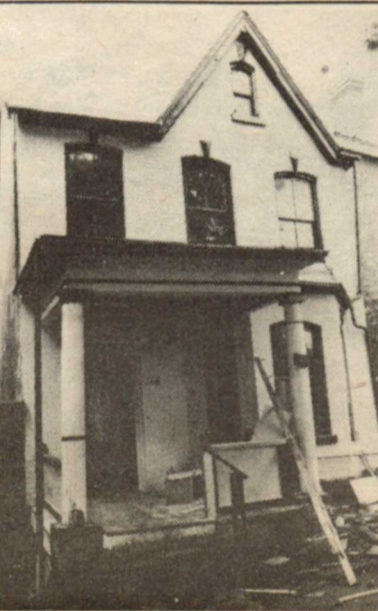
This unpretentious 9-room house on Berkeley Street will be used to house problem roomers with drinking and medical problems. Although still under repair, some roomers are expected to be moving in very shortly. Photo by Steven Evans
