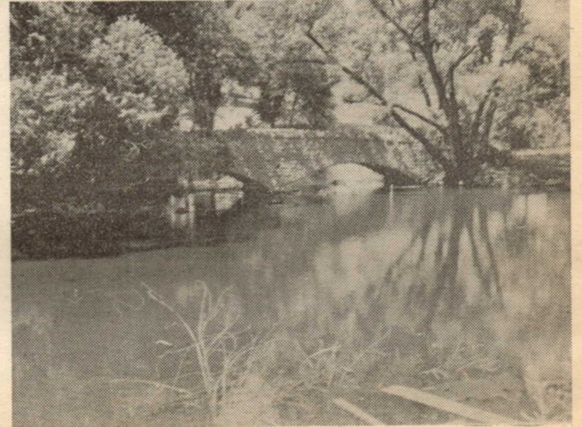
View of debris-laden pond in Riverdale Park. Photo by Steve Hooper
