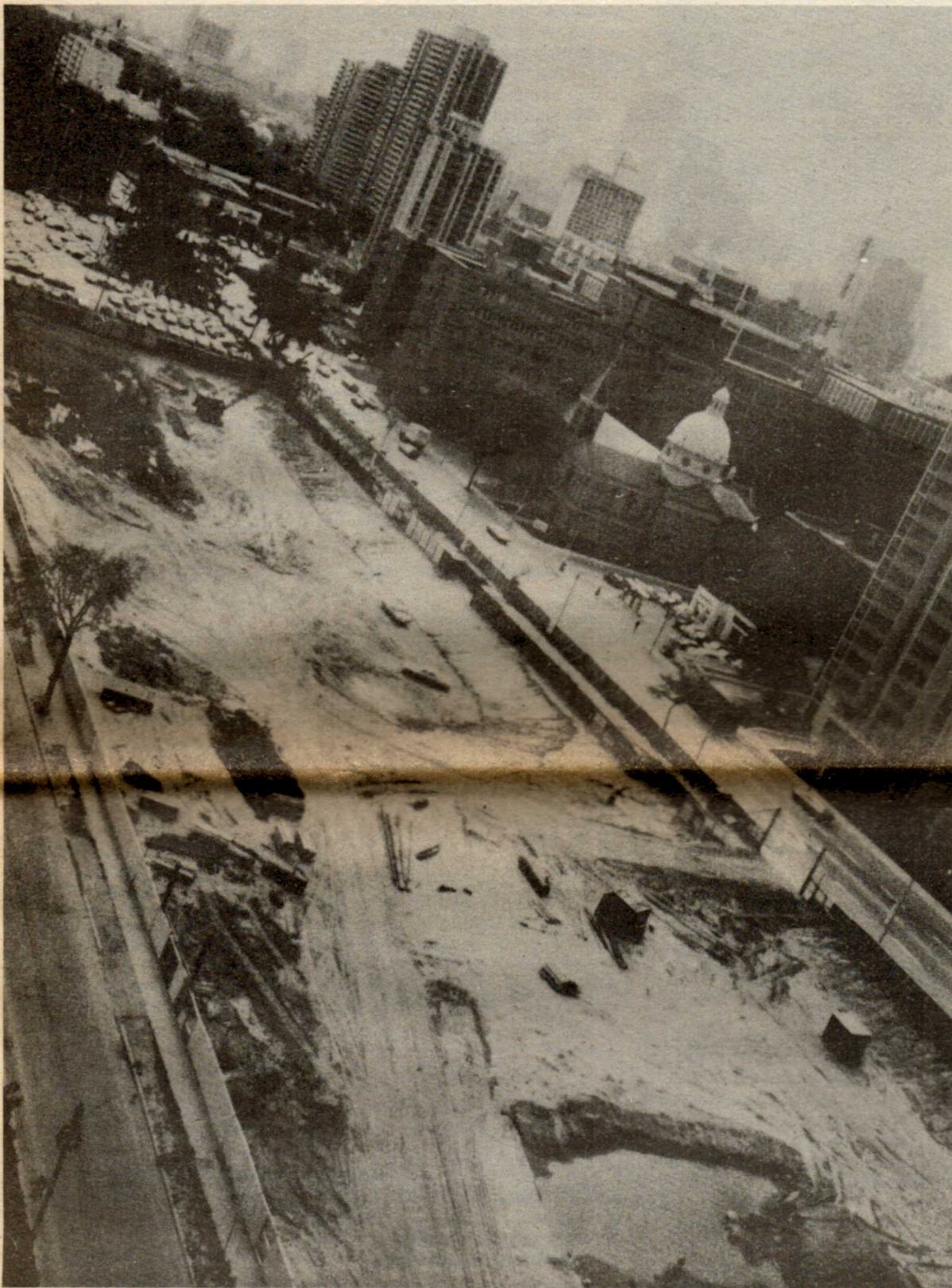
Unconfirmed reports have it that the above pictured West St Jamestown site, owned by Meridian, is up for sale. The reason given is that Meridian can't get financing to go ahead with construction. Although construction seems to be going on, some people in the area believe the activity on the site is to it being used as a park until construction money is available. Photo by David Ruppel
