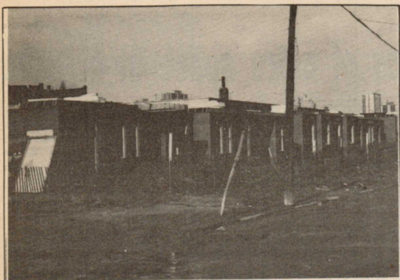
Construction is proceeding on schedule for the 17 new houses being built on Trefann street as part of Phase I of the Trefann Urban Renewal Scheme. photo: e. kolompar
