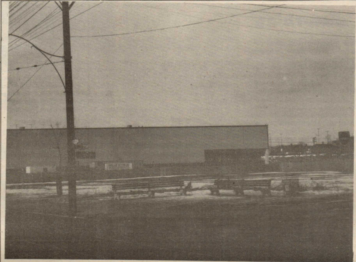
Work is progressing nicely on changing the former Dunlop site on Queen Street east near Booth to Jimmy Simpson Park. Among the structures being built is an artificial ice rink and two swimming pools. Ironically, one of the swimming pools is being built directly in the path of the proposed Scarborough Expressway.
