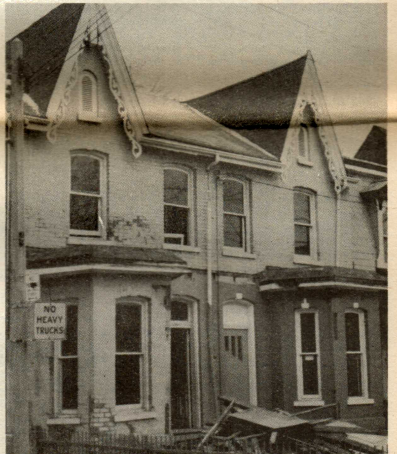
Two houses at the corner of Dermott Place and Carlton Street in Don Vale. They are presently undergoing reconstruction as part of the DACHI project.
