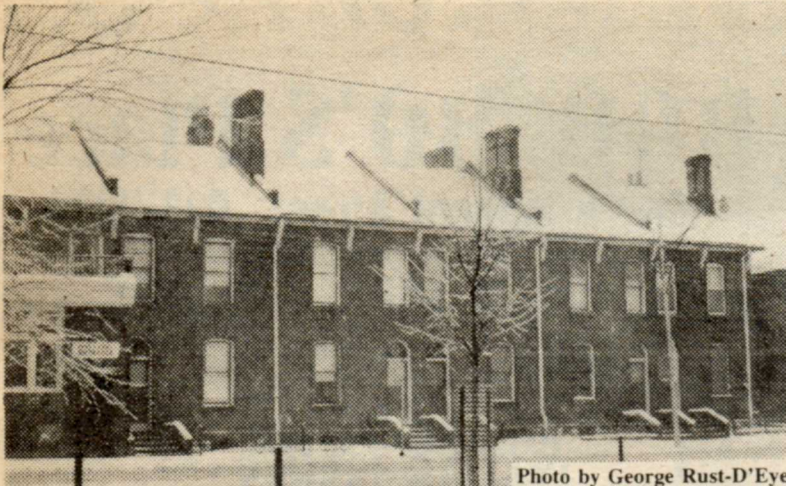
Photo by George Rust-D'Eye A very beautiful and well-proportioned terrace from the 1880s, at 436-446 Gerrard St. E. Listed by the THB.
