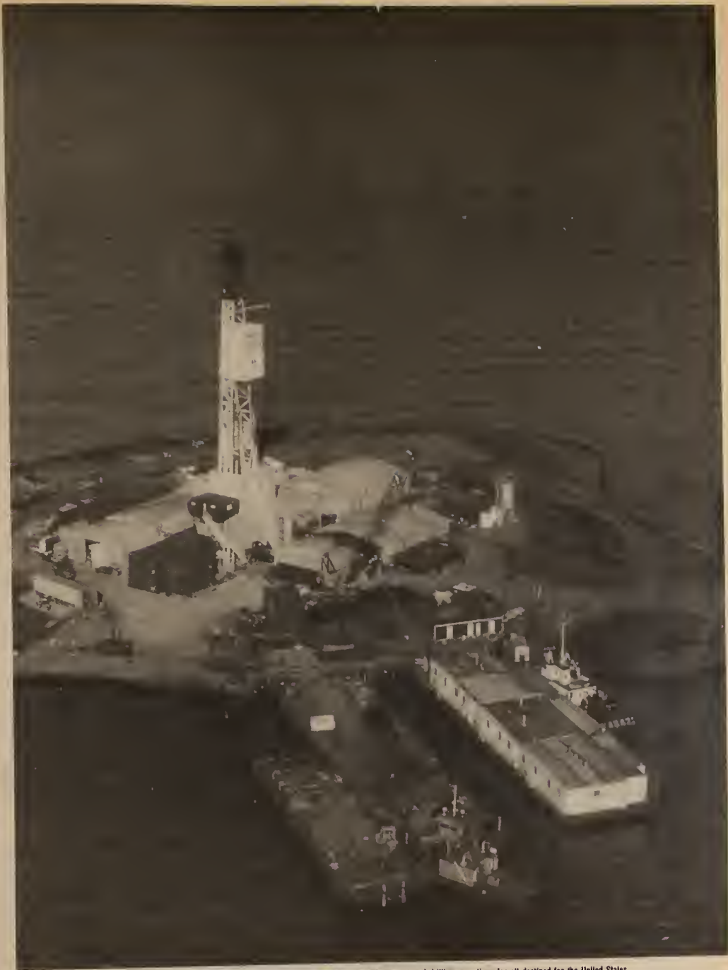
Imperial Oil's artificial island in the Beaufort Sea permits year-round drilling operations for oil destined for the United States.
