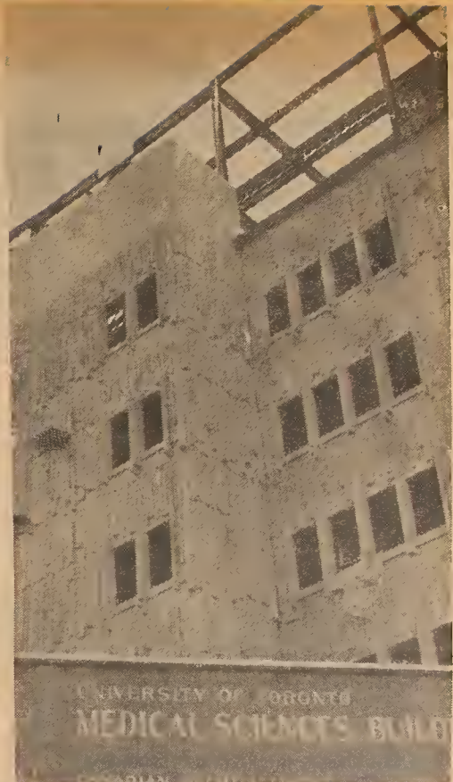
Construction of Canada's largest medical centre has been set back many months because of a strike. See Page 6. photo by JOE WEINSTOCK
