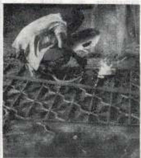
Spot welding a steel window frame in a Tanzanian worker co-op. (See story, page 17.)
