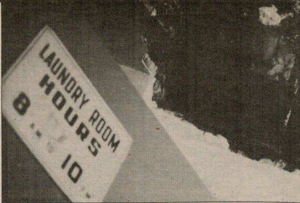
Gaping hole in ceiling at Barbara Apartments. (Photo: Ted Hebbes)
