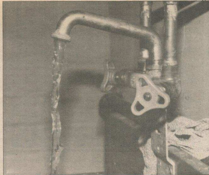
Pickering's drinking water hazardous. (Photo: David Smiley)
