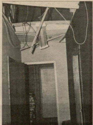
Acme Lathing's office at 73 Alness St. after the high order dynamite bombing on September 2, 1972.
