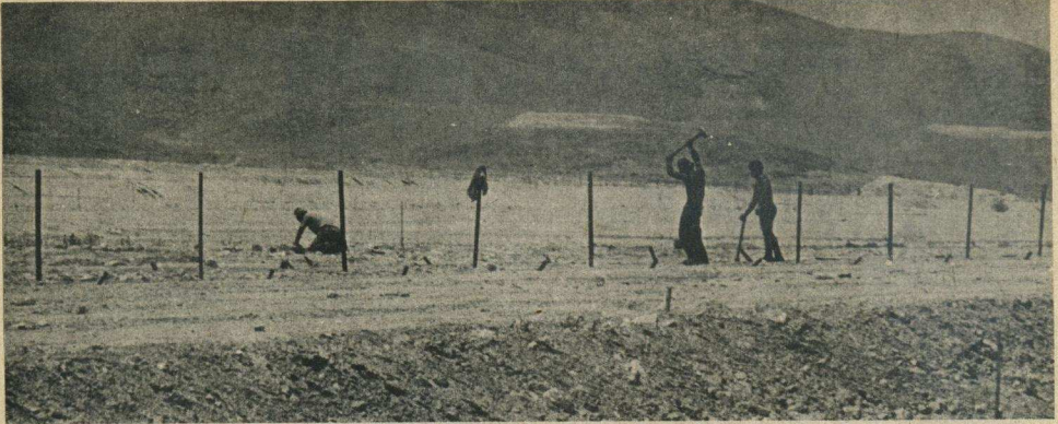
Land being levelled and fenced for new nahal (military) settlement in Jordan valley
