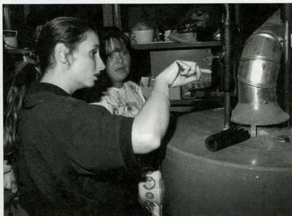
EnviroSense workers Rachel Moore and April Aikin inspect furnace in a Nepean home.
